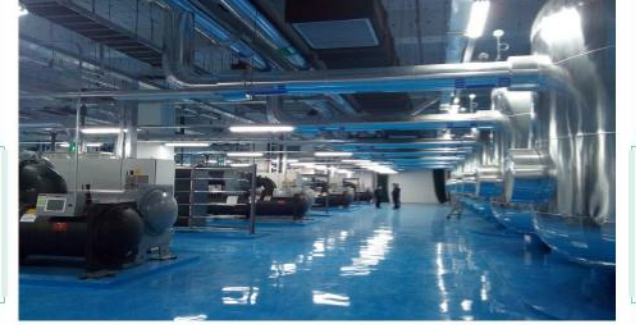
Huawei Cloud Data Center, Daqing, Heilongjiang
