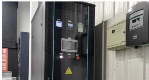
GLP Liquid Cooling Pilot Project, Changshu, Jiangsu
