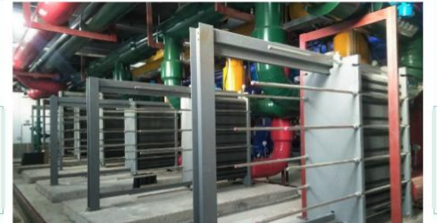
China Unicom Belt and Road Data Center, Xinjiang
