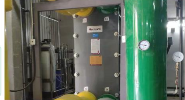
State Grid Intelligent IoT Data Center, Beijing
