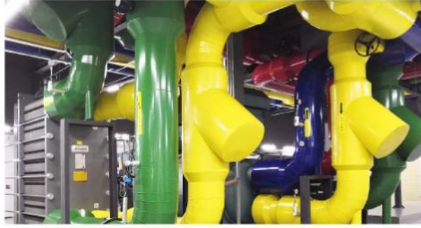
Shanghai Chengdi & Xiangjiang Lingang Intelligent Technology Innovation Industrial Park Data Center, Shanghai (ByteDance)
