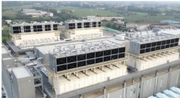
Gangcheng Intelligent Manufacturing Data Center, Suzhou, Jiangsu
