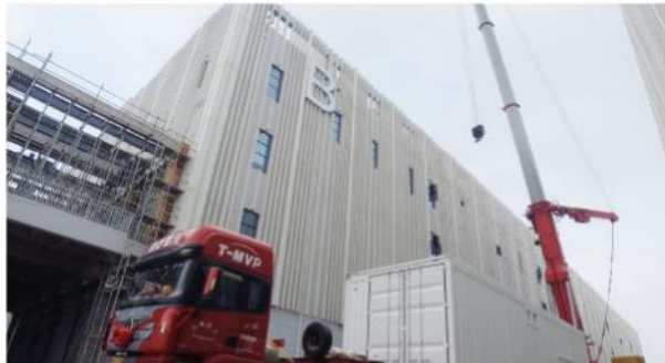
GLP Changshu Sanyi Data Center Phase II, Jiangsu (Tencent)
