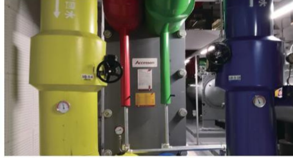
Beijing City Cloud Data Center, Beijing
