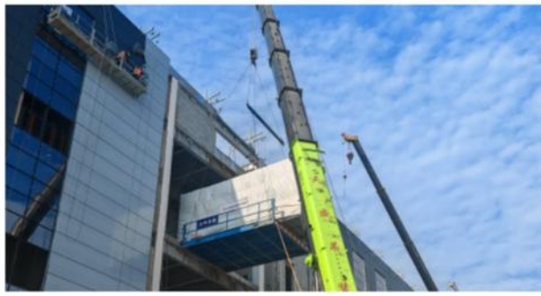
XX Cloud Data Center, Wuhu, Anhui
