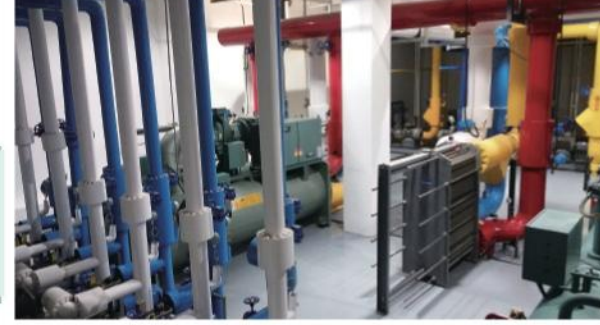
China Telecom Cloud Computing Base, Qingdao, Shandong
