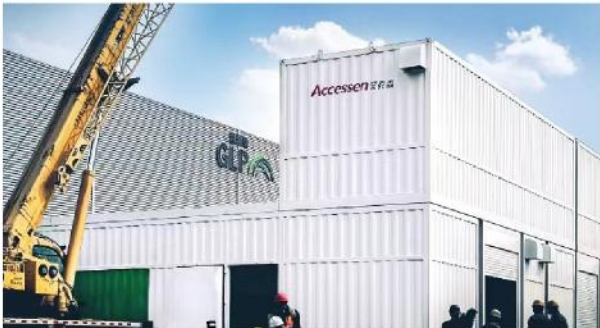
GLP Changshu Southeast Data Center, Jiangsu
