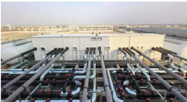
GLP Changshu Sanyi Data Center Phase I, Jiangsu (Tencent)
