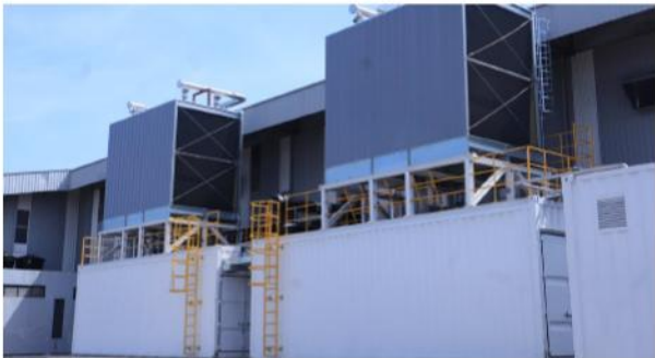
XX Data Center, Penang, Malaysia
